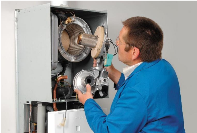
Image 4: Regular servicing and automatic flow balancing to optimize the system are essential for maximizing heating savings.
